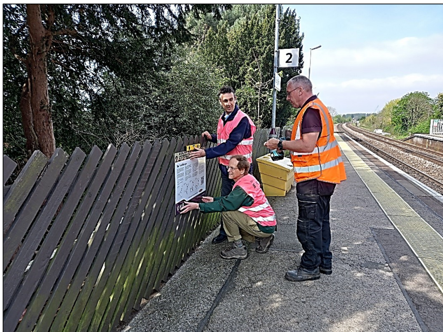
Fixing one of the boards; note typical Midland Railway diagonally slatted fencing.
